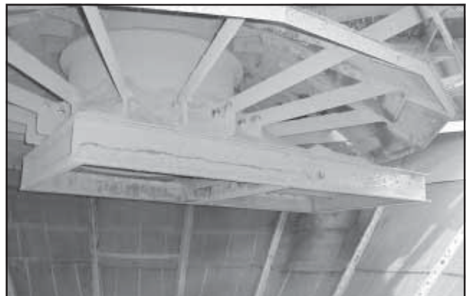
5-C. Bypass Gate and Shed after it has been in operation.
