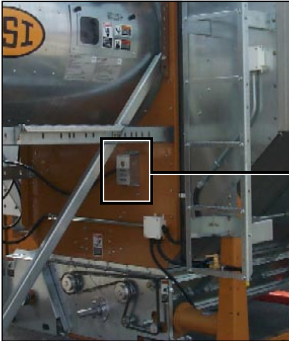
Air Switch location.
