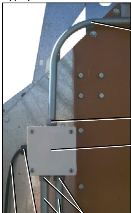
Upper junction box.
